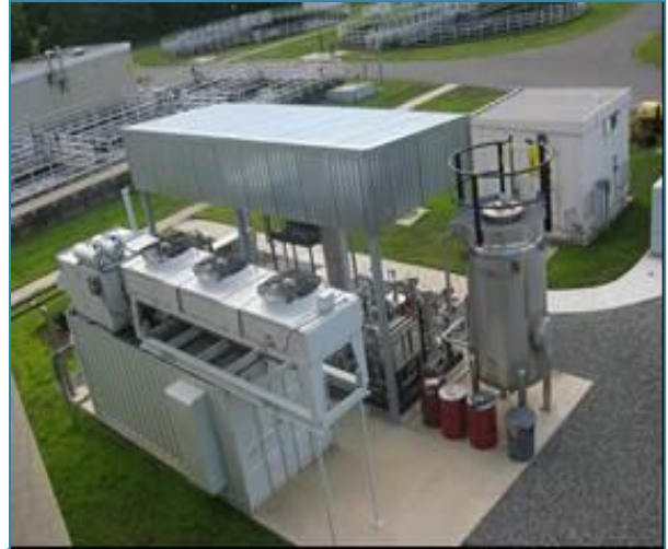
Technology: Anaerobic Digesters, Combined Heat and Power by 240 kW Engine/Generator and 50.4 kW Solar Field.
